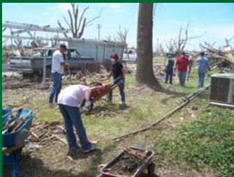
Removing debris in Greensburg, Kansas after a monster tornado.
